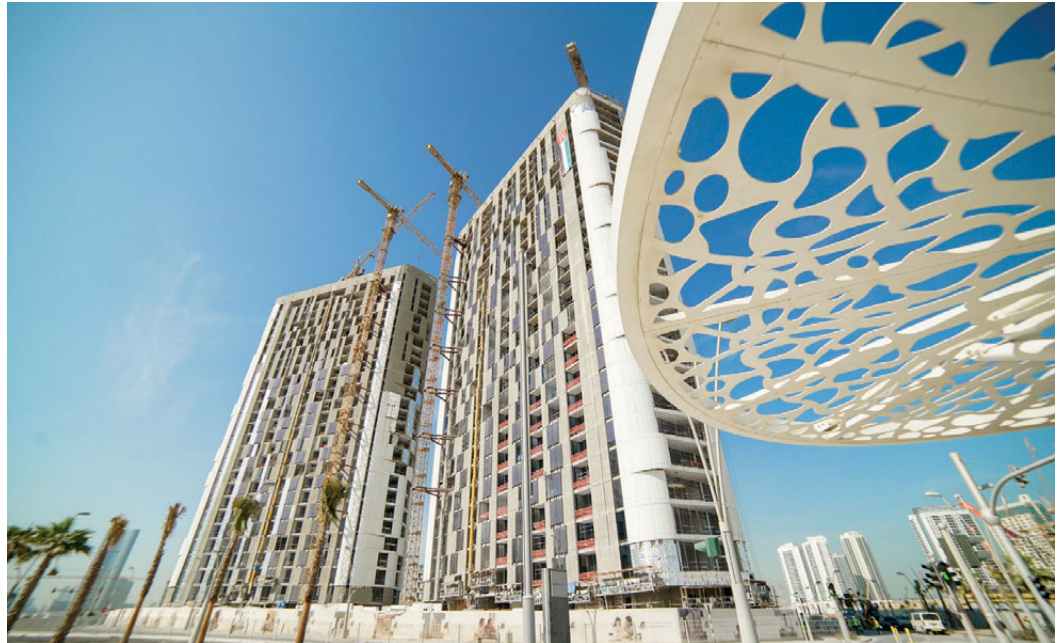
Glazing and façade work on Aldar’s Meera, a two-tower project on Reem Island in Abu Dhabi, is nearing completion.
